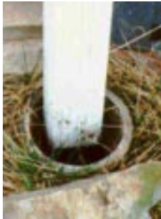
Improperly connected downspout
